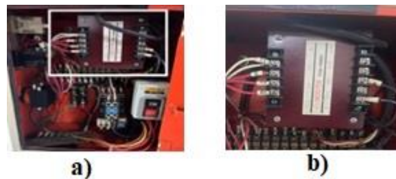
Figure 6. a,) Control wire of grinding machine connection before b) Control wire connection after
